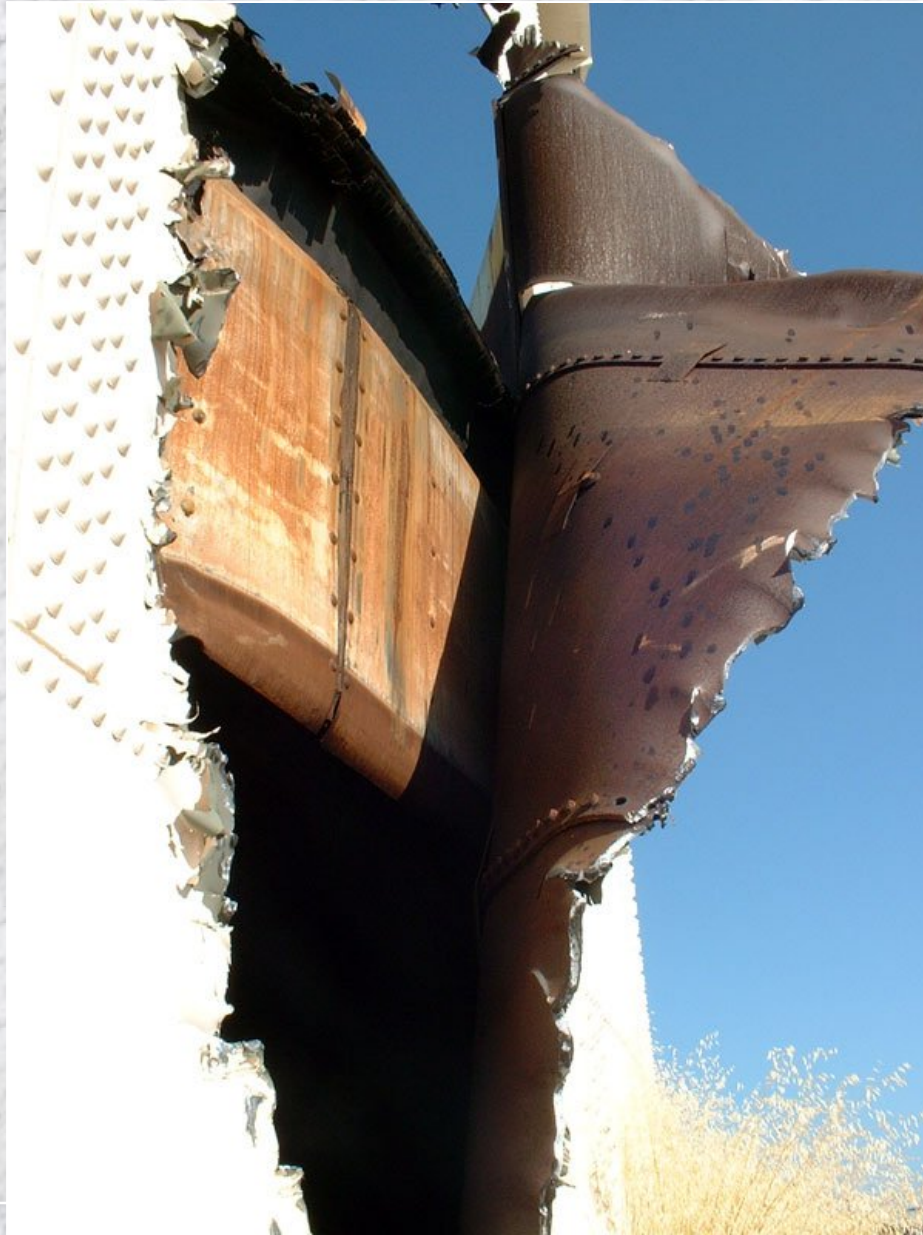
FIGURE 3 – FLOATING ROOF INSIDE OF TANK
