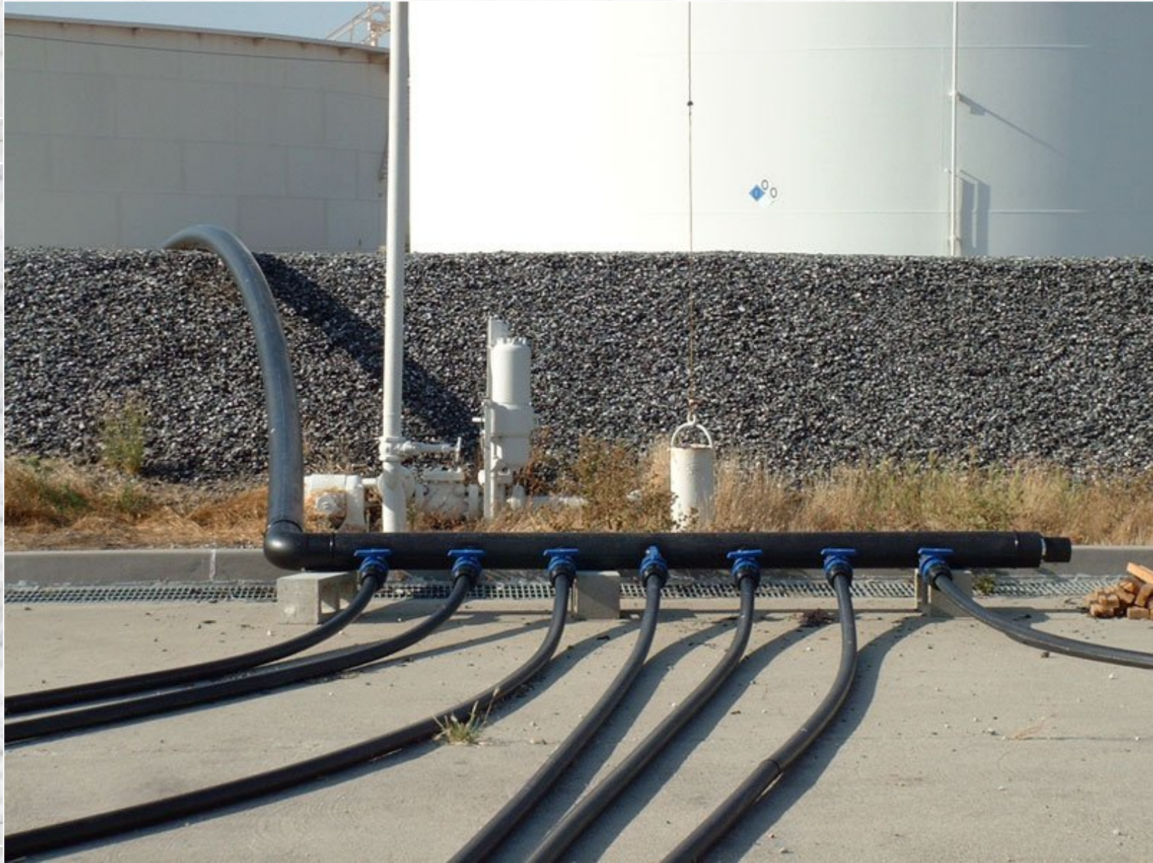
FIGURE 2 – TRUCK FIELD STAND MANIFOLD
