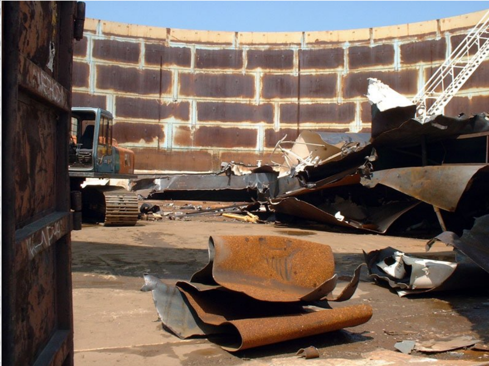
FIGURE 4 – FLOATING ROOFTOP DEBRIS
